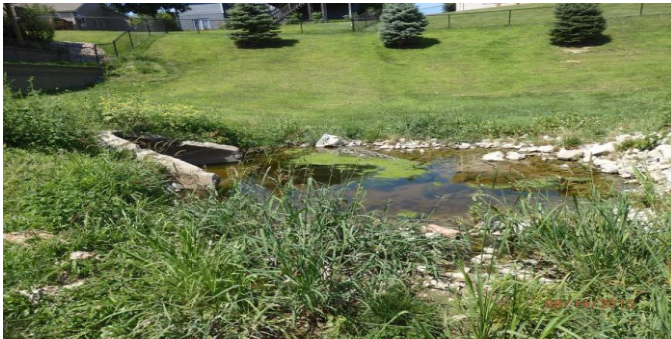
South Pond - Collapsed Inlet
