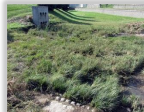
Figure 5.2 – Wet basin grass & weeds around Briarwood inlet
