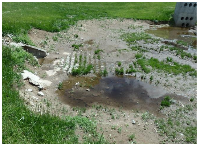
Figure 3 – May 2019; Standing Water near the Briarwood Drive Outlet/Basin
