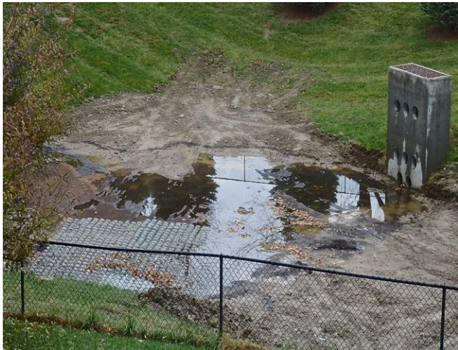
Figure 1 - November 2018; Standing water near outlet
