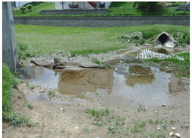
Figure 2 – May 2019; Damaged Turf Reinforcement Matting (TRM)
