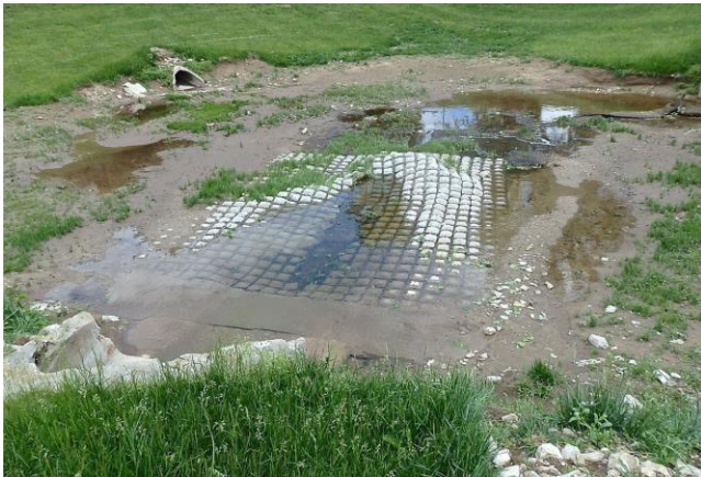
Figure 4 – May 2019; Flexamat Damage caused by spring downpour
